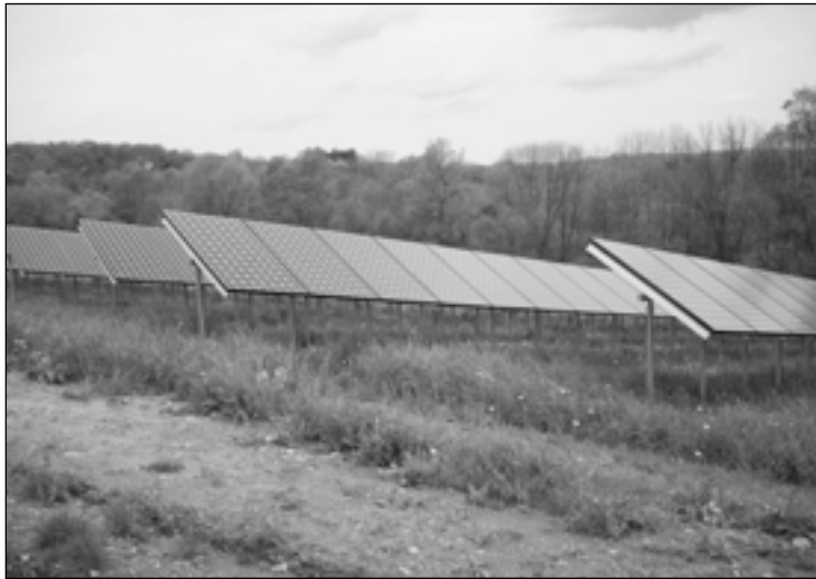
These solar panels stand along the eastern side of the Timex Group building. In all, 800 panels generate 285,439 kilowatt-hours of energy a year. (Cristina Commendatore photos)
